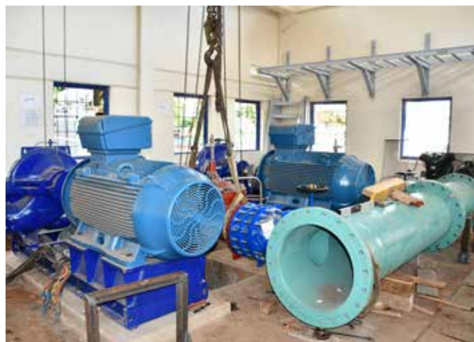
Ongoing improvement of Kabete Water Treatment Works that include installation of new water pumps (Credit Kibet Cheptumo/KNA)
